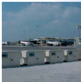
4 Apojet units, Malpensa Airport, Italy
