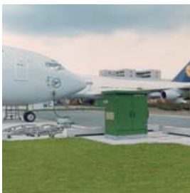
Ground power equipment, Frankfurt Airport, Germany
