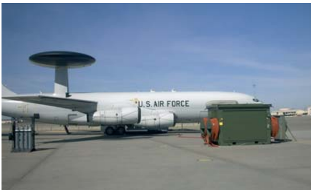
Piller equipment at AWACS bases worldwide
