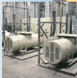
Piller central systems, SeaTac Airport, USA
